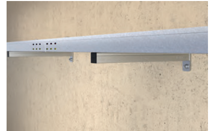
Cable tray on cantilever arm
